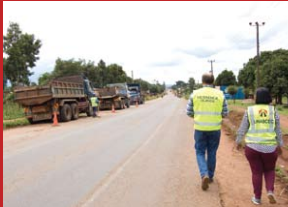
Maintenance works on Tororo- Mbale-Soroti Road by Mota-Engil Engenharia E Construcao Africa S.A.
